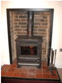
The woodburning stove in situ
