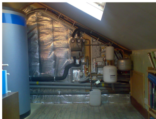
Solar water heating system and cylinder in loft
